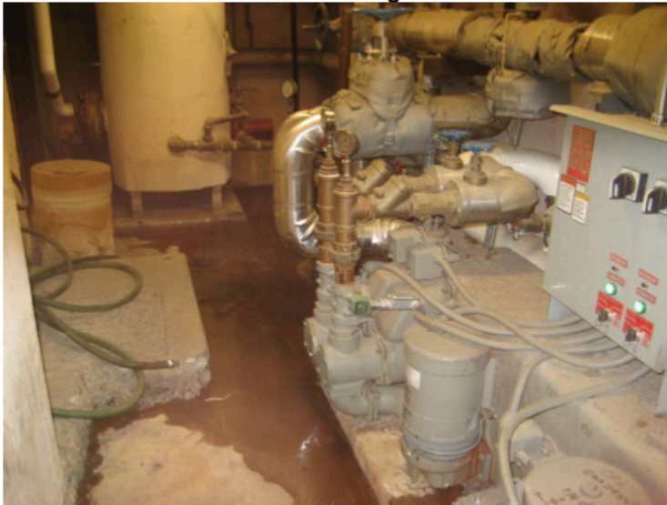
Figure 3-7 Condensate flowing to drain
