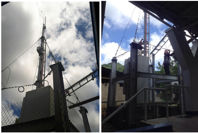
Figure 1. The cell tower site in San Andres, where the experiment was conducted. The VSAT and power equipment are housed in the large metal box at bottom, the BTS is mounted midway, and the antenna is visible at the top of the tower.
